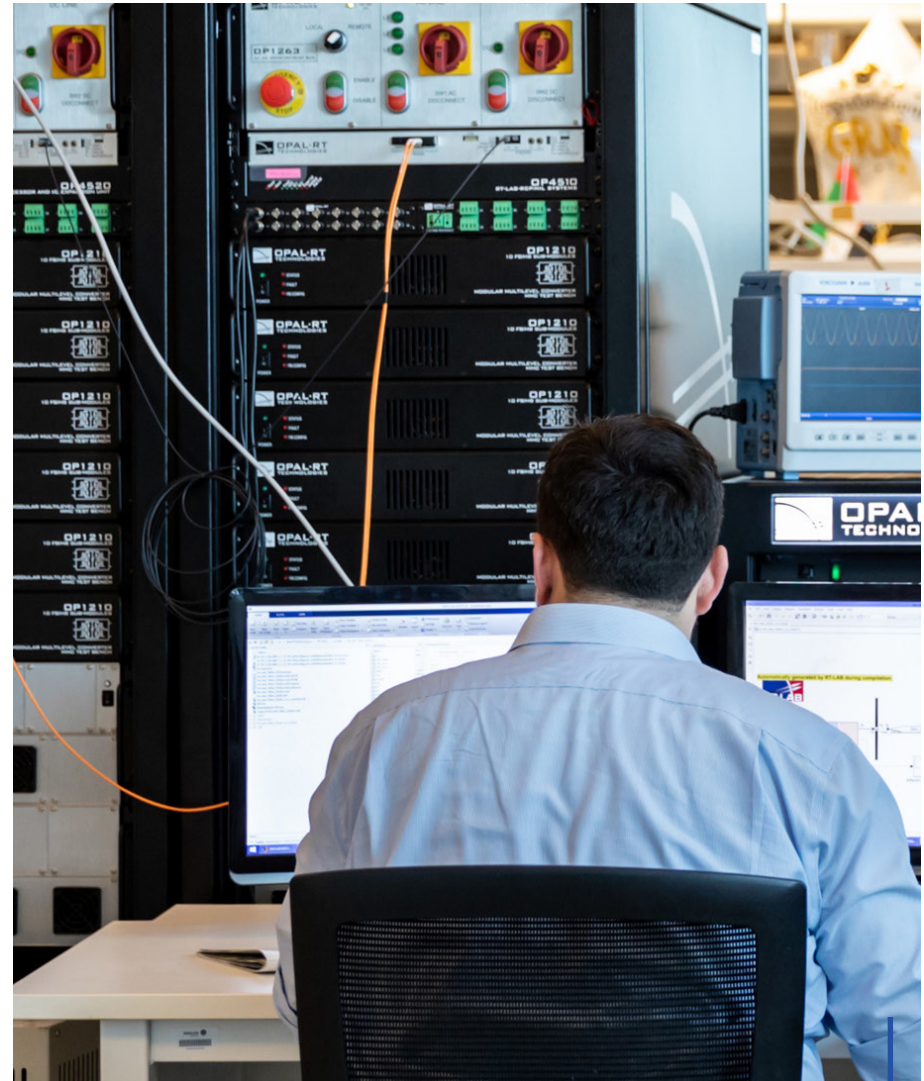
Advanced Power and Energy Center (APEC)
